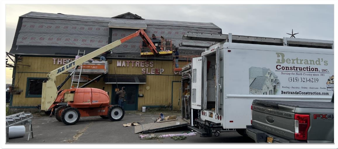
Construction underway at the future home of the Bent Beam Brewery in Canton
