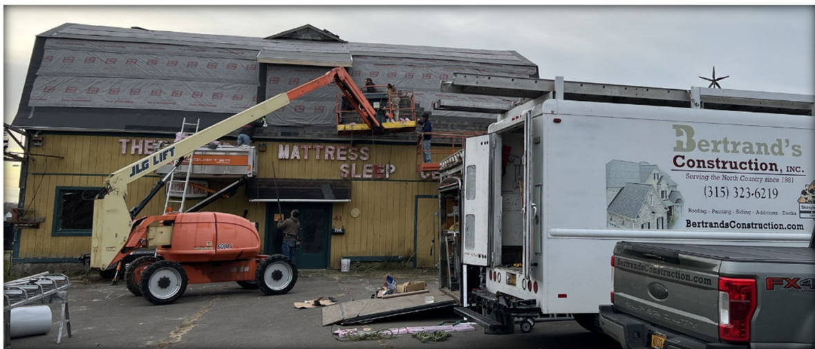
Construction underway at the future home of the Bent Beam Brewery in Canton
